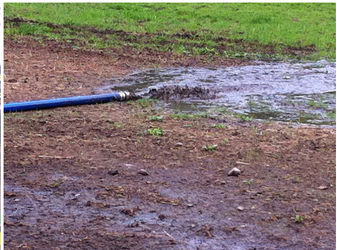
Sediment and debris discharging
