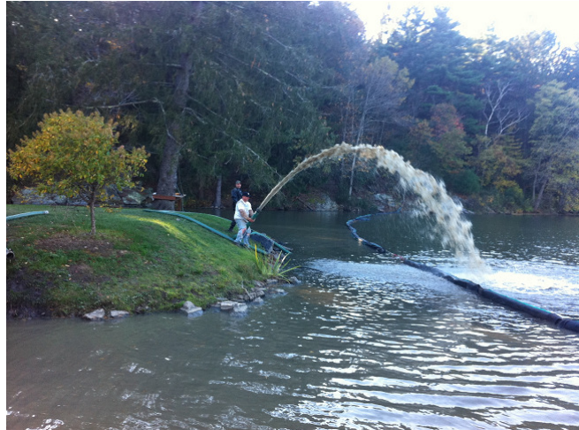
4" Discharge with 400' of Hose
